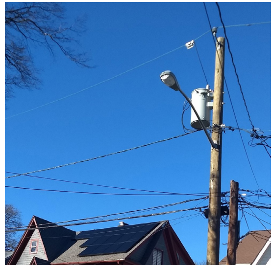
Updated Power Pole and Transformer to Increase Capacity for Solar and Electric HVAC
