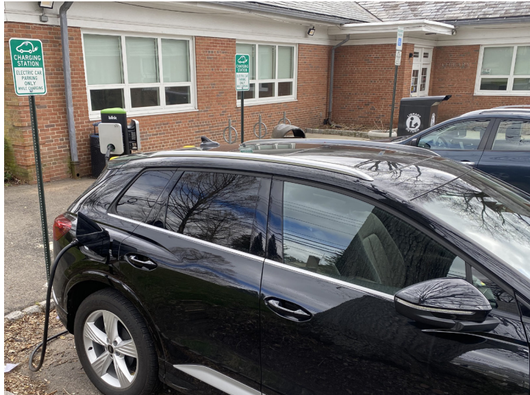
Electric Vehicle Charger at the Maplewood Library Hilton Branch
