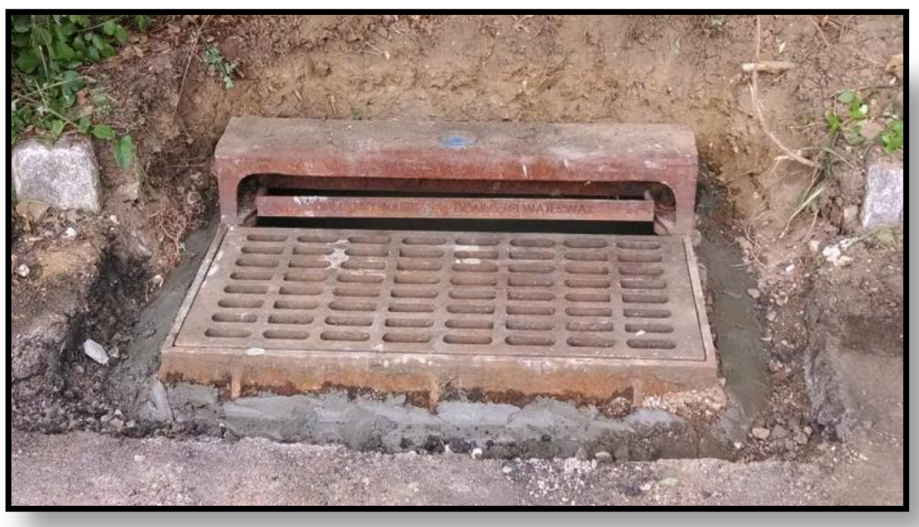
Stormwater Inlet Retrofit with Eco-Safe Bar and Bicycle Safe Grate
